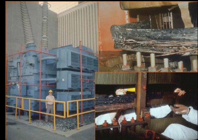
Damaged transformer by GIC (USA)
